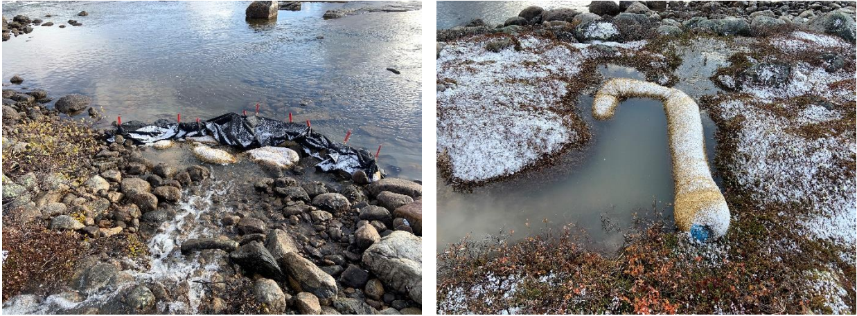
Figure 3 Sediment barriers and retention booms (straw) positioned downstream of the sedimentation/decanting systems at the construction site
