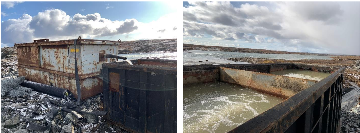
Figure 1 Sedimentation/decanting systems for water generated by excavation work at the construction site
